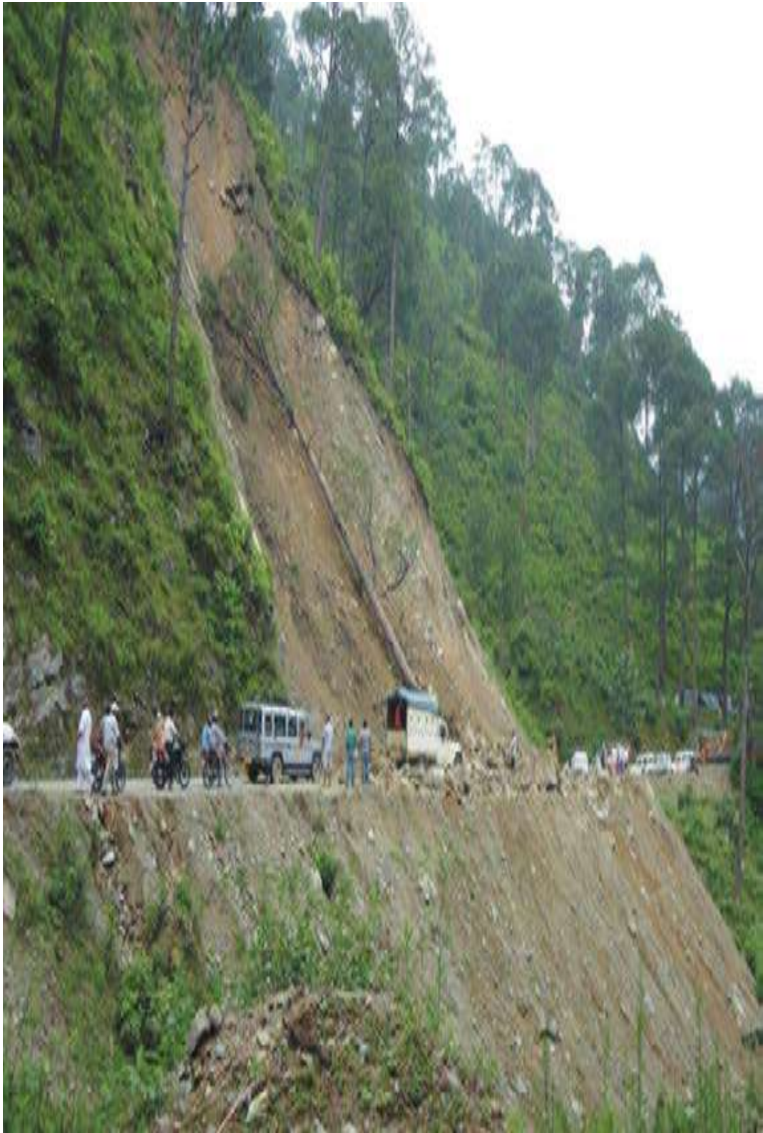
Figure No: 2 Landslides in Rudraprayag - Guptkashi road
